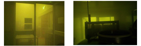
Image 2a & b – The Chlorine dioxide gas inside the penicillin manufacturing plant during remediation.
